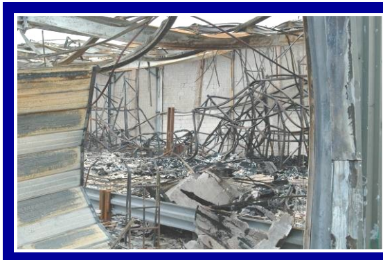
Fire Damaged Steel Framed Warehouse
